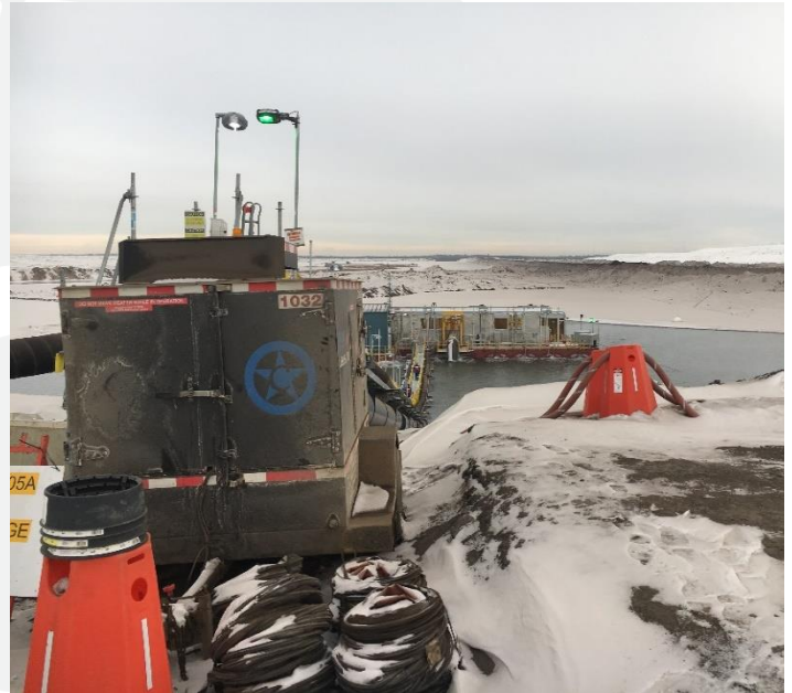
A CH15HS heater delivering hot air to a tailings barge from 500 feet away
